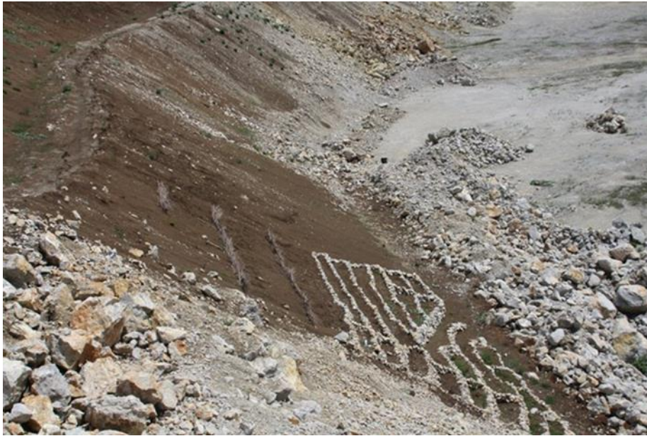
Figure 8.6 Amass of plant and rockfill material to form terraces on a high slope
